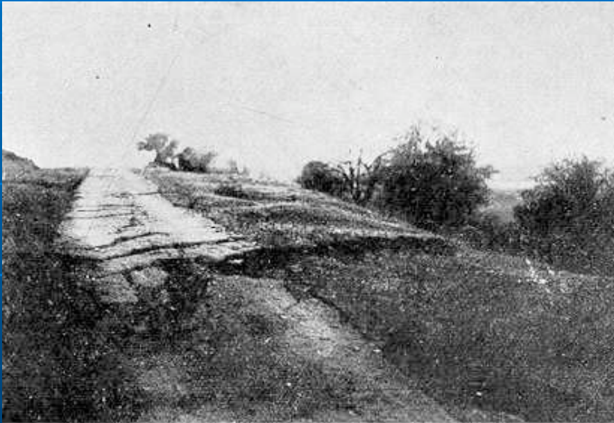
Subsidence of the Tsarigrad road near Papazli village.
